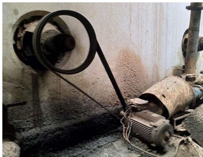
Figure 2: View of current agitator system installed at factory
